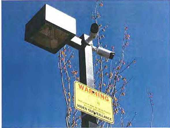
G City Park Security Camera Installation Project
