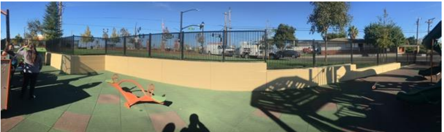
Photo of the Wall
